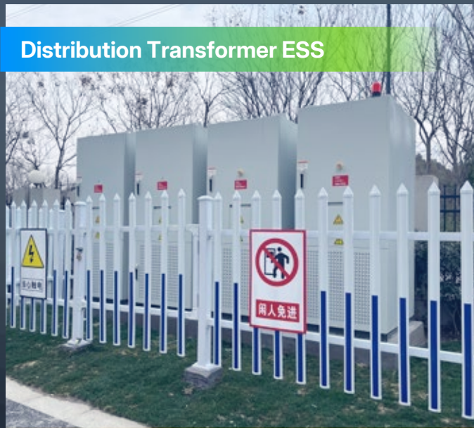
Location: Chengdu Capacity: 400 kW / 860 kWh Product: HoyUltra series Scenario: Factory Highlights: Three-phase balancing, overload mitigation
